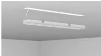
3. Connecting AC wires
